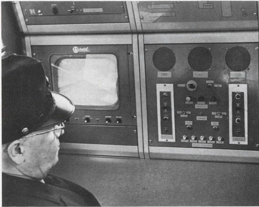
Central control station monitors strategic points in a plant. In this Honeywell system, television scans an outside gate and sensitive sonic detectors guard the interior. The console includes fire detection and alarm equipment.
