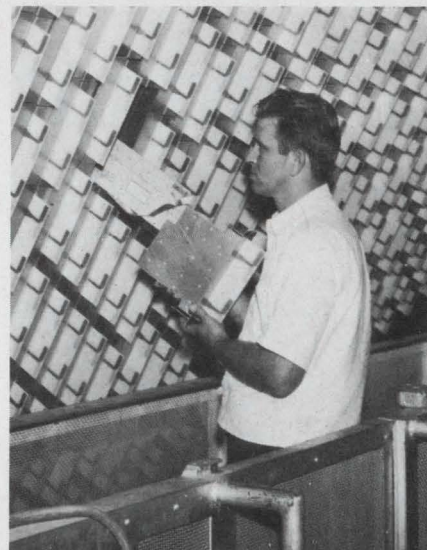
A phase-shifter module is installed in the collecting side of the large microwave lens in the new radar.
