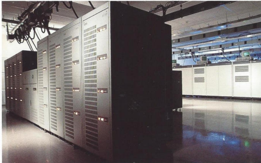
A modular approach to data center design, grouping equipment by type, makes for a more efficient and productive working environment.
